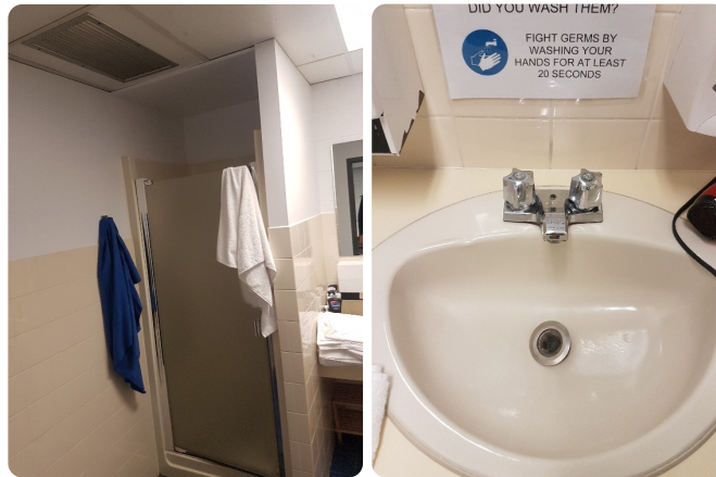
Figure 3.8.1-3: Fitness Center washroom water fixtures
