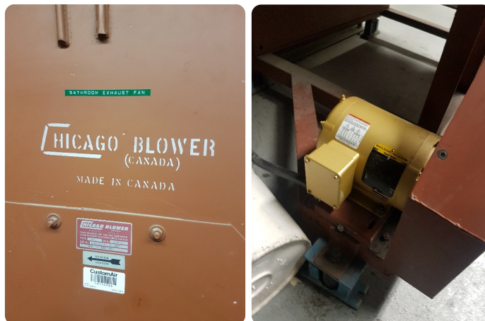
Figure 3.3.4-1: Washroom exhaust fan: casing (left) and motor (right)
