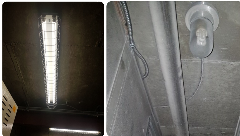
Figure 3.2-8: Service area lighting: elevator machine room (left), and inside AHU1 (right)
