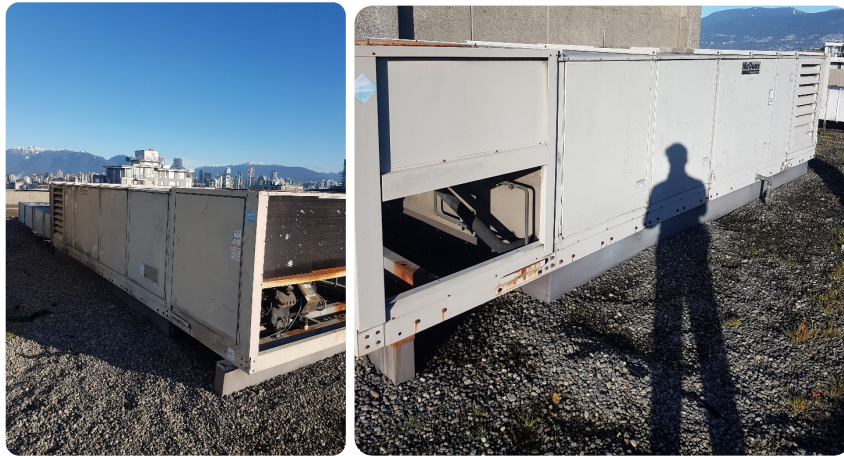
Figure 3.3.2-1: AHU2 front view (left), and AHU2 side view (right)
