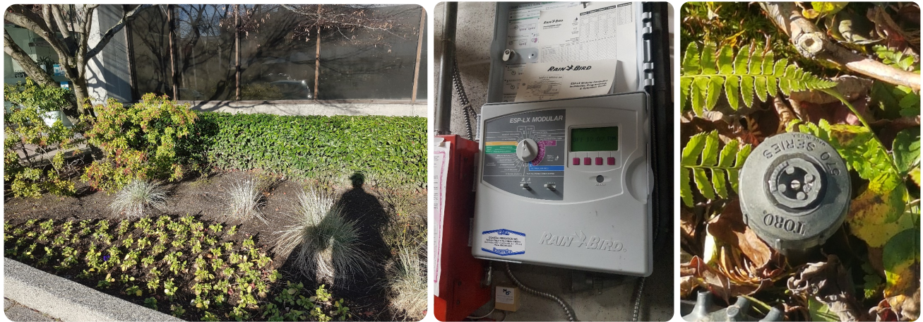
Figure 3.8.3-1: Irrigation System: general (left), controller (centre), and sprinkler (right)
