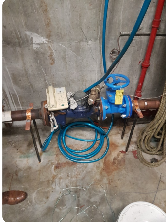
Figure 3.8.1-1: Main building water meter
