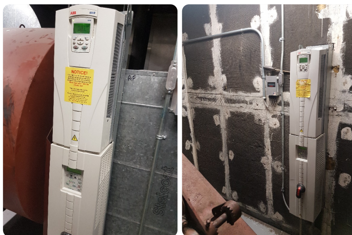
Figure 3.3.1-2: AHU1 return fan VFD (left), AHU1 supply fan VFD (right)
