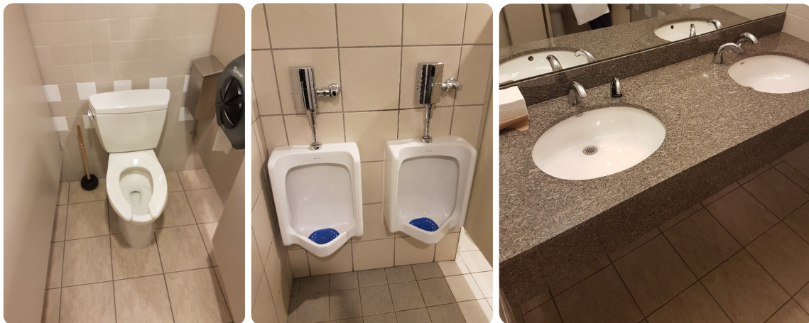
Figure 3.8.1-2: Office washroom water fixtures: toilet (left), urinals (centre), and sinks (right)
