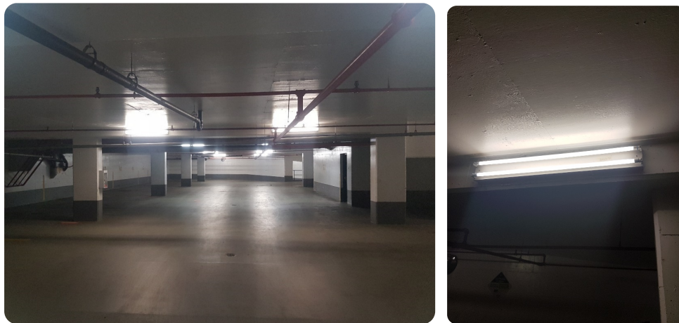
Figure 3.2-10: Underground parking lighting: general (left) and LED lamps (right)
