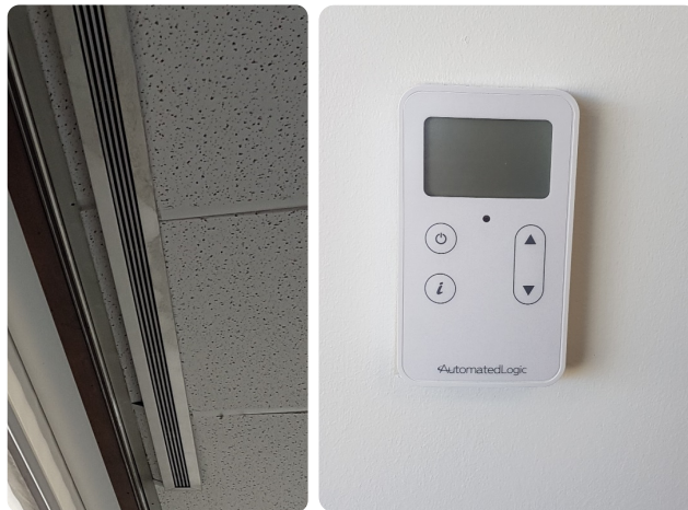
Figure 3.3.3-1: Typical FCU distribution vent (left) and typical DDC thermostat (right)
